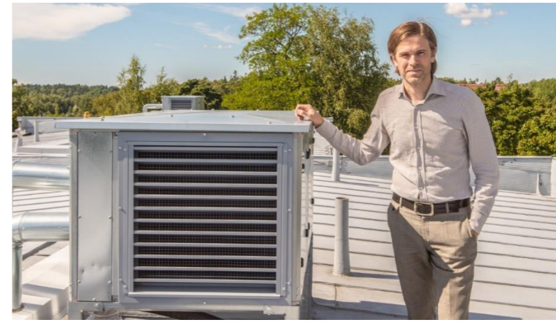
or One exhaust Heat Pump in one apartment house
